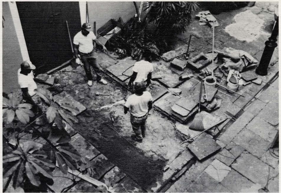
Renovation and maintenance work continued throughout the spring as the Collection prepared for the annual meeting of the American Association of Museums, held in New Orleans in June. Shown above are workmen laying flagstones, part of the process of leveling the central courtyard. Photo by Jan White Brantley
